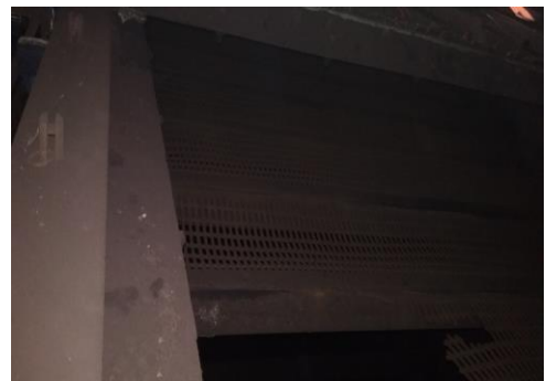
Fig 2.3. Damaged screen of screen house
