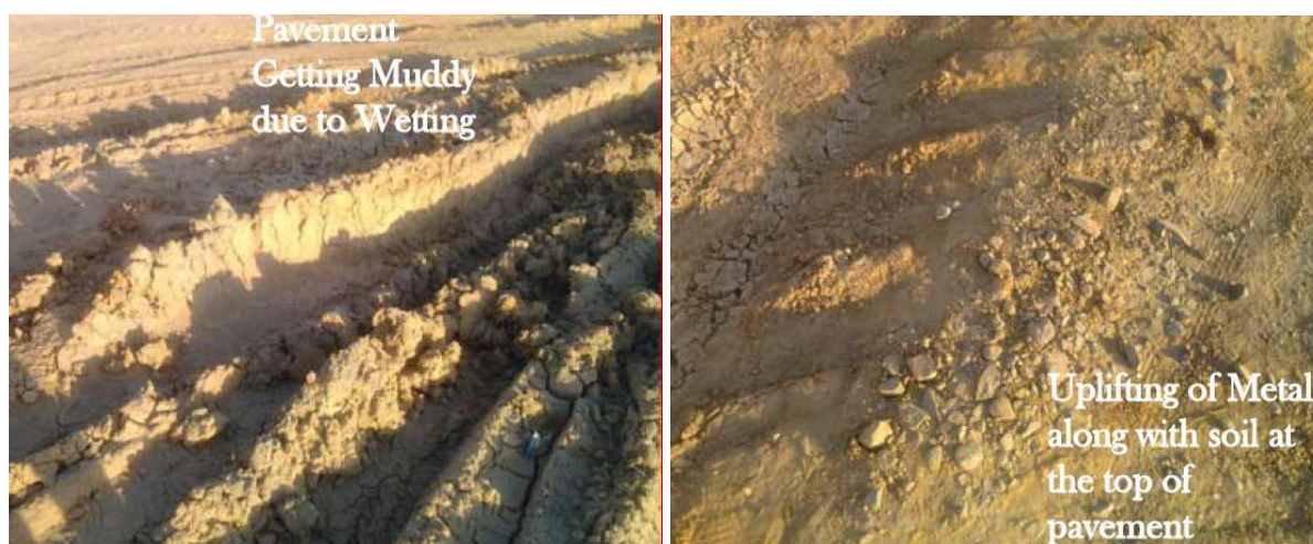
Fig. Existing Deformed Pavement at BKT Factory, Bhuj
