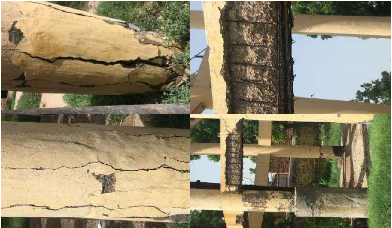
Figure-4.2 Field Structure Exposed to Aggressive Exposure Condition
