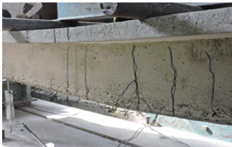
Figure 6. Failure of girder before Retrofitting
