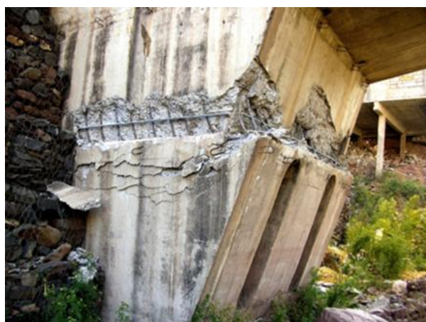
Figure 1. Shear failure of abutment at cold joint of Garhi Dupatta Bridge.
