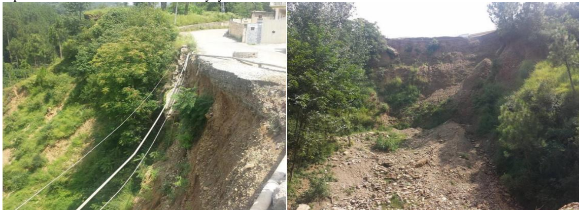
Figure 1-1: Slope Failure View
