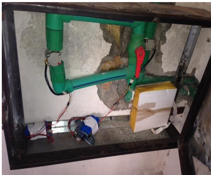
Fig: 02 Flow Meter installation and Data
