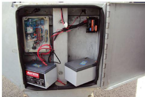
Fig. 6. LCC old control housing box [12].
