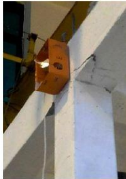
(Fig 3.4 Material failure)
