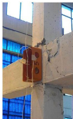
(Fig 3.3 Shear force region cracking)
