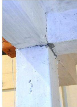
(Fig 3.1 Vulnerable beam column joint)
