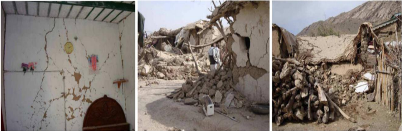
Figure 1.1. Observed damage mechanisms during 2008 Baluchistan Earthquake: In plane shear cracks in wall (Left), in plane cracks and corner failure (Middle), collapse (Right). (N. Ahmad,2011)
