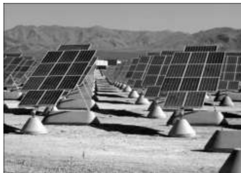
Fig.8 Unit of PV Array
