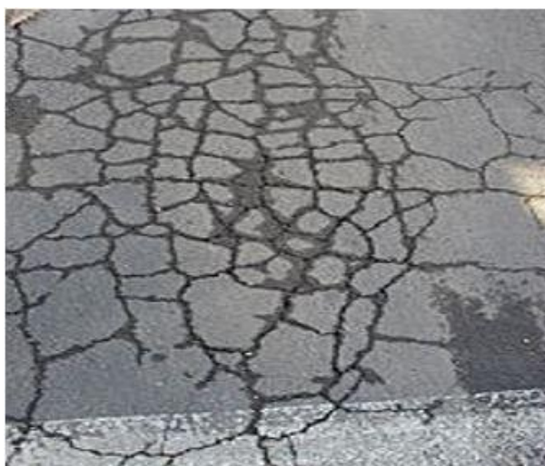
Figure 1. Crocodile pattern cracking
