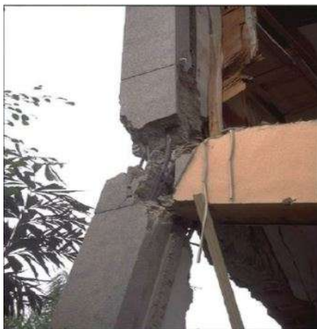
Figure 1. 1999 Chi-Chi Earthquake (Taiwan)
