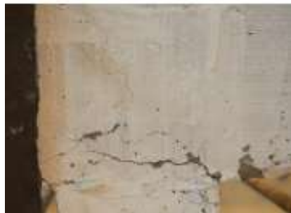
Figure 6. Cracks in the beam-column joint area
