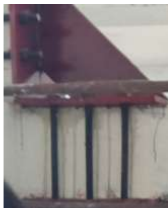
Figure 7. Observance of flexural cracks in the beam
