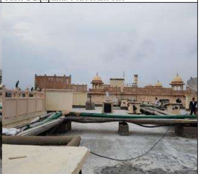
Photo-4 Piping Arrangements on Mother Slab Rear View
