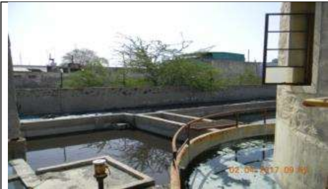
P1 Corroded Element at Site
