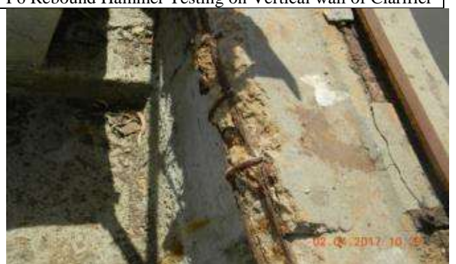
P8 Exposed Main & Secondary Rebar without cover
