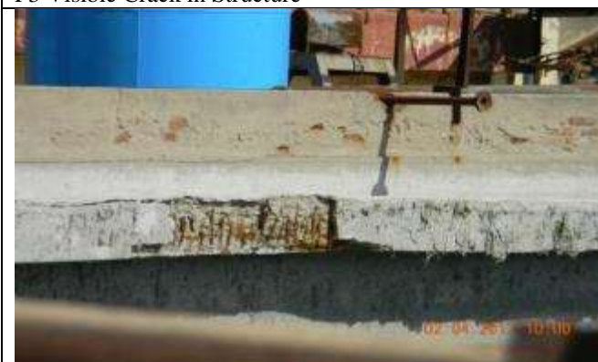
P5 Exposed Beam Reinforcement
