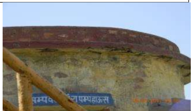
P4 Exposed Reinforcement at Pump House
