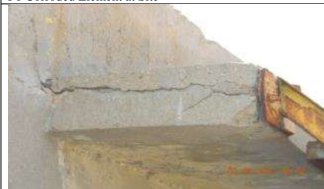
P3 Visible Crack in Structure
