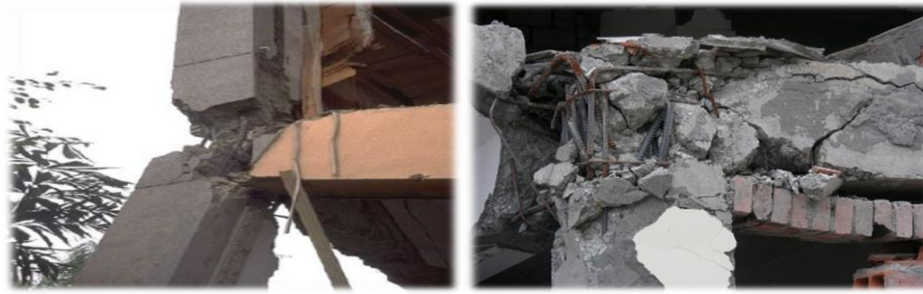
Figure 2: 1999 Chi-Chi Earthquake (Taiwan) Figure 3: Wenchuan earthquake 2008 Insufficient confinement in the joint
