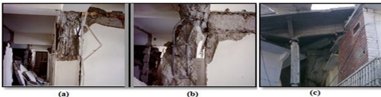
Figure 1: Damaged beam column joints
