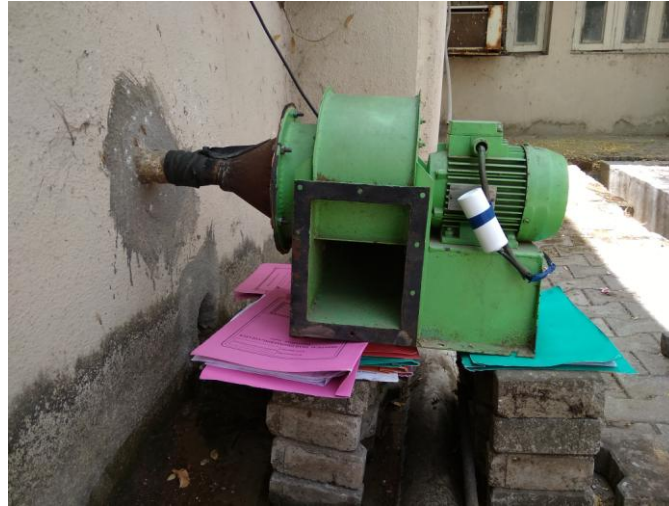
“Figure 2. Suction Blower at exhaust”
