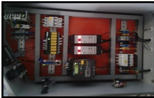
Fig. NO. (9) Actual image of Control Panel
