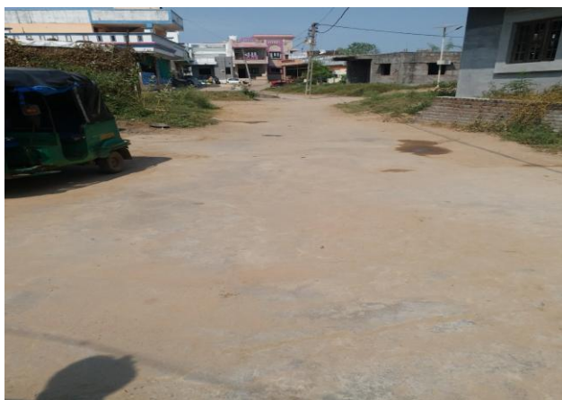
Fig- Road Condition
