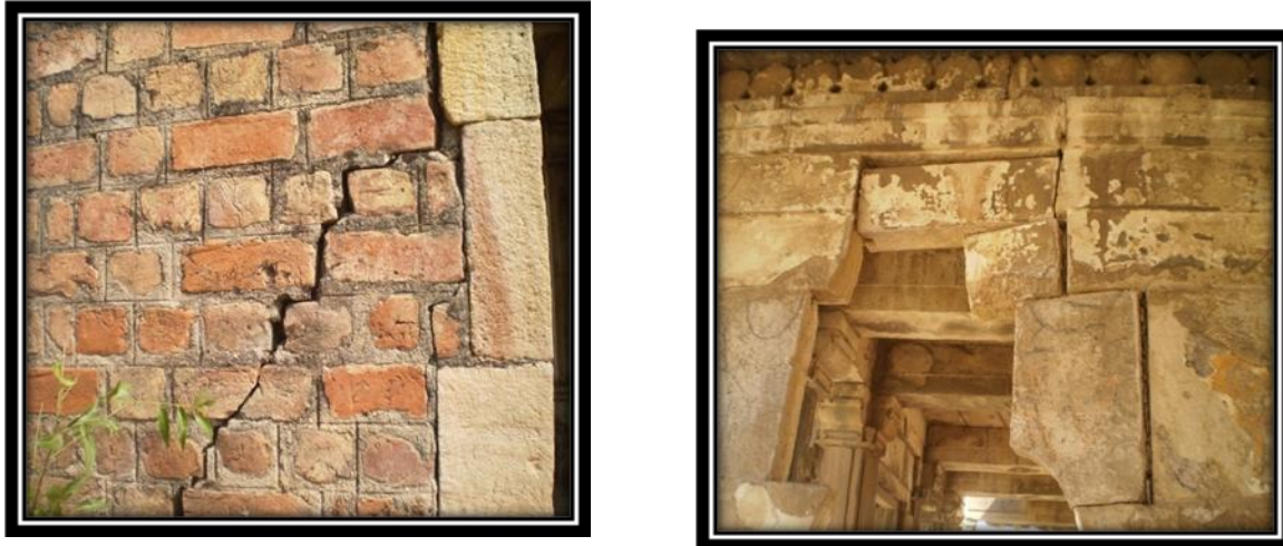
Figure 3.2 : Damages found in sarkhej Roja [12]
