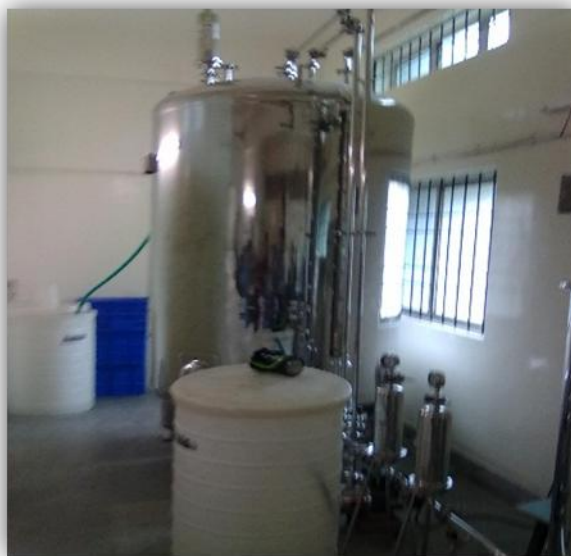
Figure 5. Stirred tank installed at Beacon Diagnostics Pvt. Ltd, Navsari
